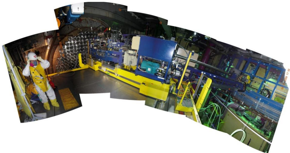
Fig. 10 Equipment for the removal of pressure tubes and calandria mounted on the pressure tube and calandria platform removal
